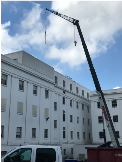
Building maintenance at Central Office is an ongoing project at ADOL. A couple of projects are pictured: The front terrace being retiled and one of the AC cooling units being replaced.
